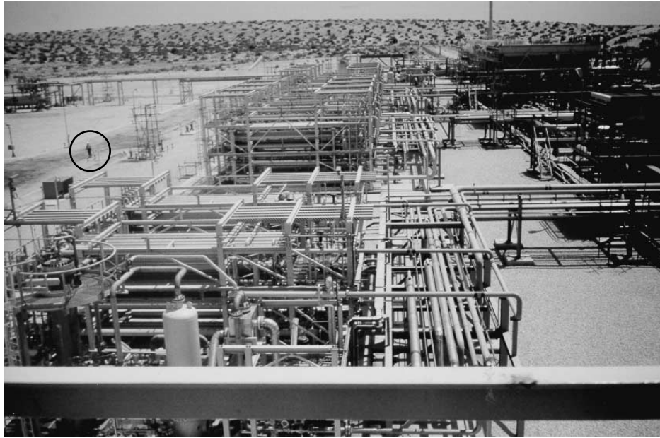
Figure 19 Qadirpur Membrane System
